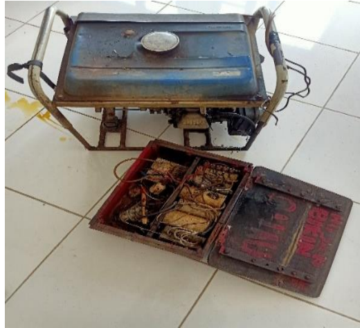
Figure 3 – Evidence of the generator and its circuit
